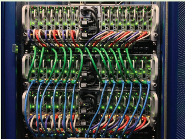
MicroCloud’s Rear Cabling Simplicity
