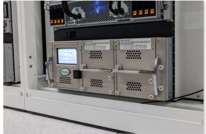
XAI Colossus Data Center Supermicro CDU On the Bottom Of The Rack
