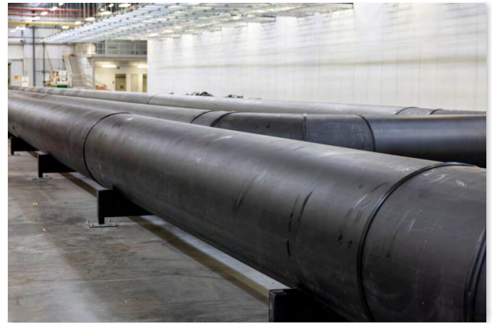
XAI Colossus Data Center Facility Water Pipes
