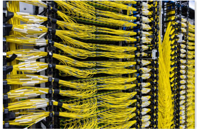
XAI Colossus Data Center Switch Fiber 1
