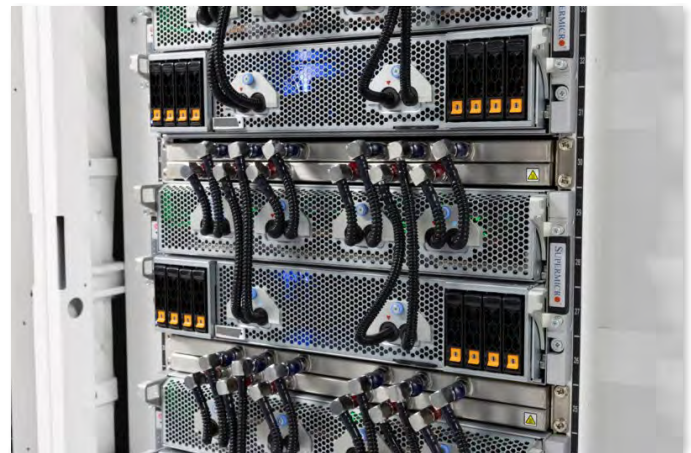
XAI Colossus Data Center Supermicro 4U Universal GPU Liquid Cooled Server Close
