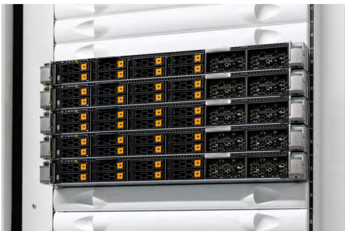
XAI Colossus Data Center Supermicro 1U NVMe Storage Node 2
