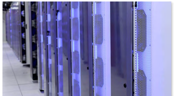
XAI Data Center Tour Rear Door Heat Exchanger
