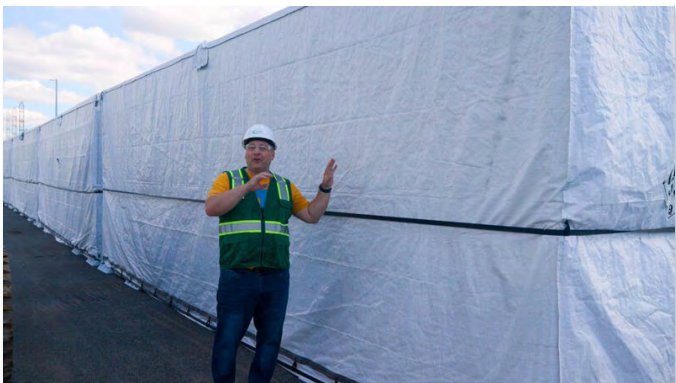
Tesla Megapacks Ready For Installation At XAI Colossus
