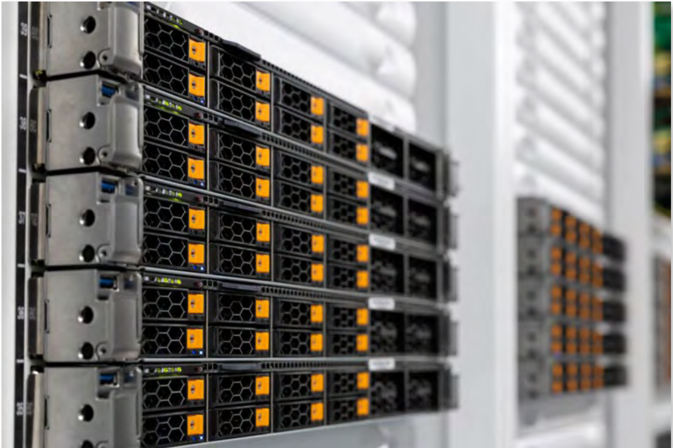
XAI Colossus Data Center Supermicro 1U NVMe Storage Node
