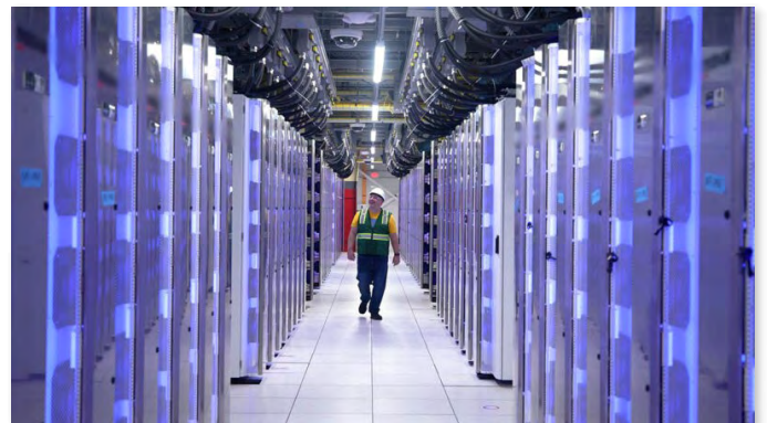
XAI Data Center Tour Rear Door Heat Exchangers
