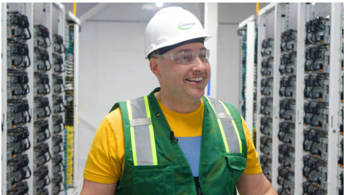
xAI Data Center Tour Patrick In Compute Hall
