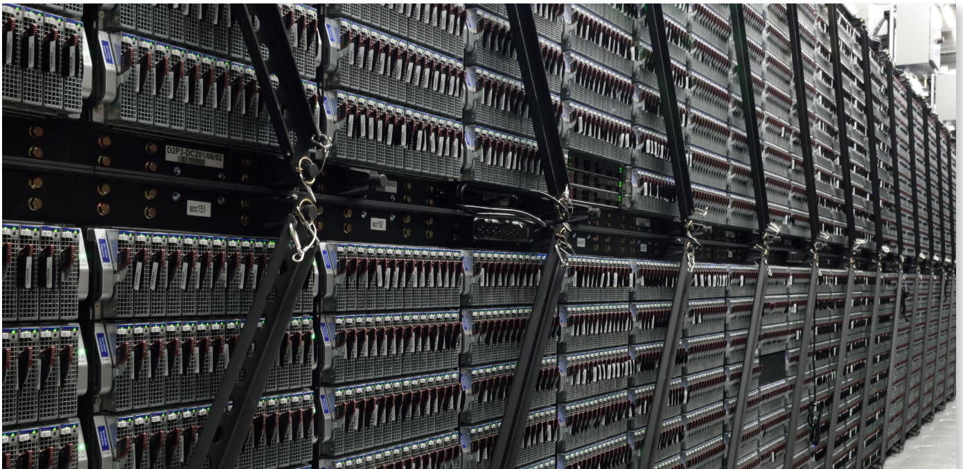
Figure 7. MicroBlade systems Inside the Data Center of the Fortune 100 company
