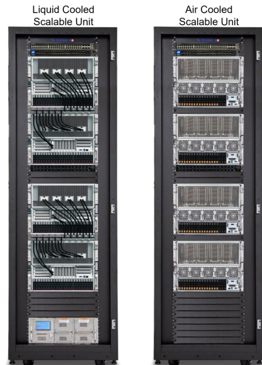
Figure 1- Liquid Cooled or Air Cooled Supermicro 8U Servers with NVIDIA H100 GPUs
